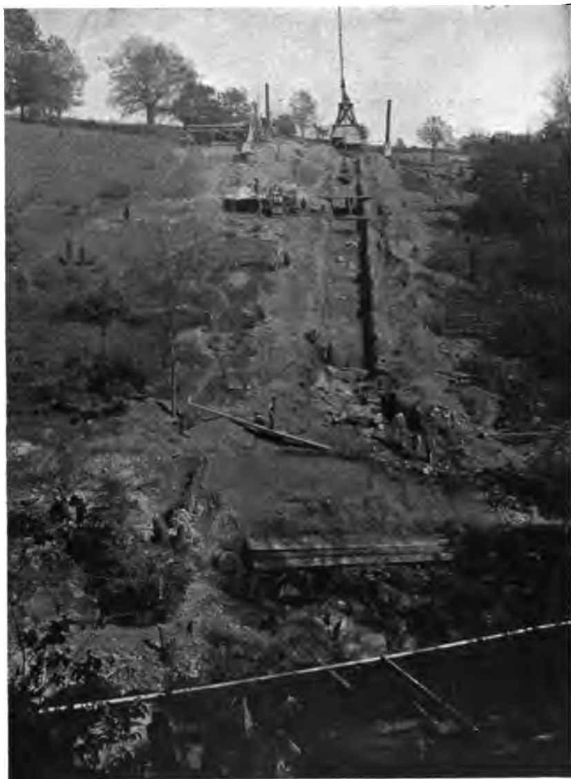
PLATE 151. —Contract 62. Indian Brook Siphon. Excavation of trench for pipe on steep side hill using cableway and grab bracket.
